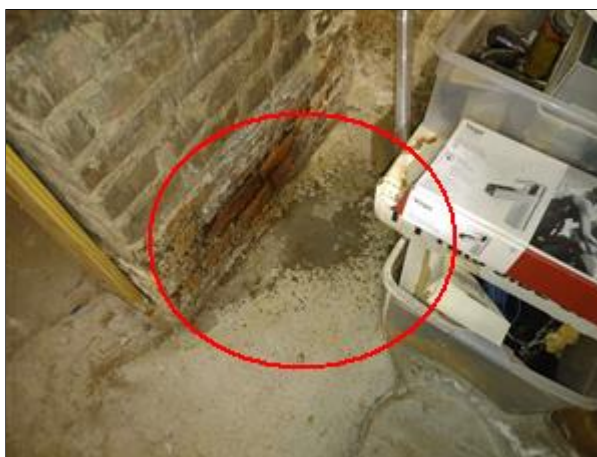
A. Picture 3 Leaks
