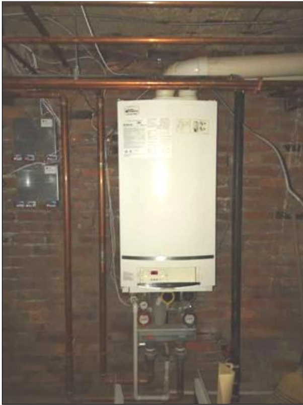
D. Picture 1 Boiler / Instant-Hot Water Heater
