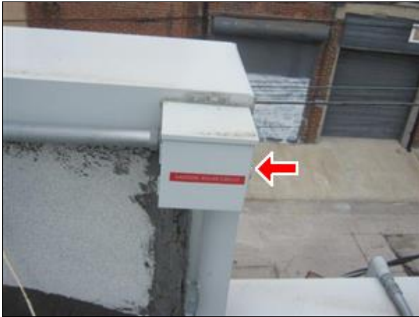
E. Picture 4 Wiring Box on Roof
