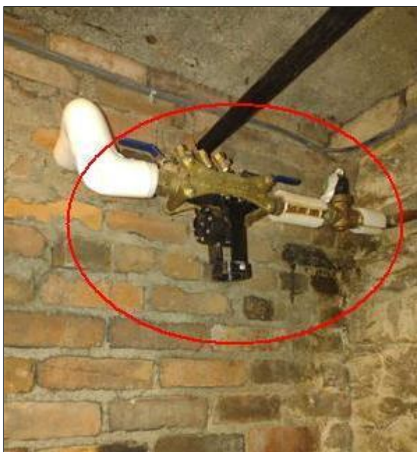
A. Picture 2 Backflow Prevention
