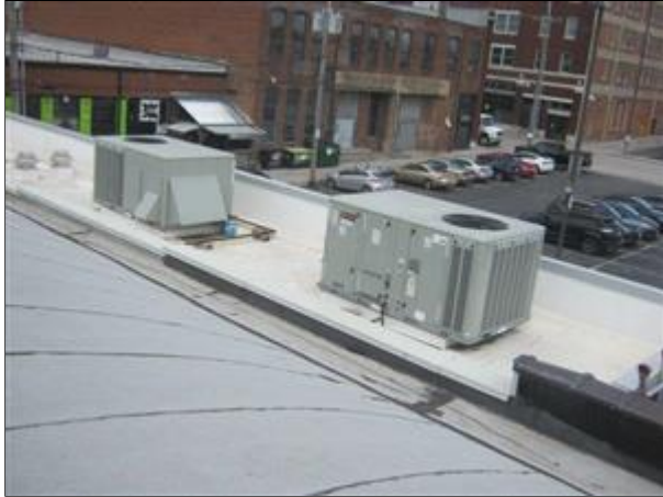
F. Picture 1 RTU / Pkg Units
