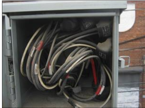
E. Picture 5 Wiring Box on Roof
