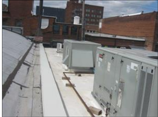
F. Picture 2 RTU / Pkg Units
