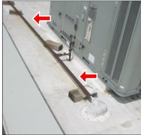
F. Picture 7 Rusty Gas Lines
