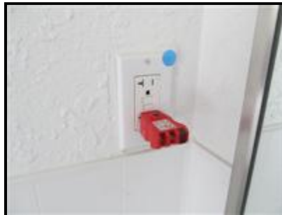
1.3 Picture 1 No Power
