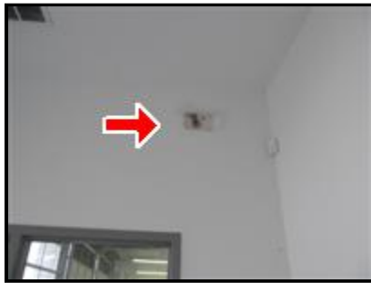
3.2 Picture 1 Missing Fixture/ Office
