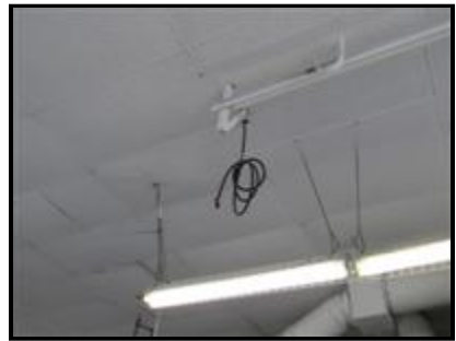
3.2 Picture 3 Shop/Capped Off Wires
