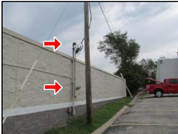
3.0 Courtesy View Of Main Electrical Entry.
