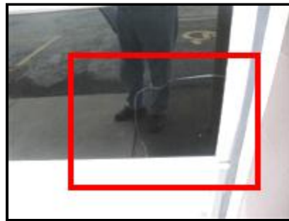
10.2 Picture 5 Cracked Glass
