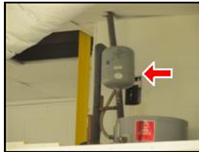
2.0 Picture 3 Expansion Tank
