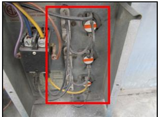
4.1 Picture 6 Strip Heaters
