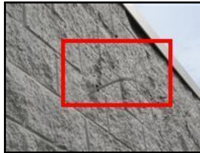
3.2 Picture 10 Exposed Wires Outside
