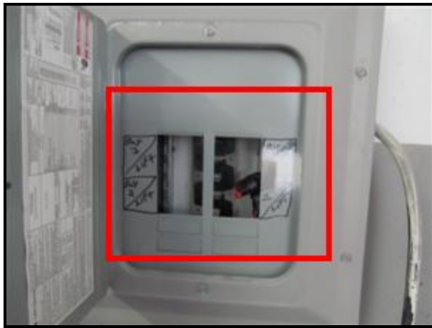
3.1 Picture 2 Open Gaps/No Breakers
