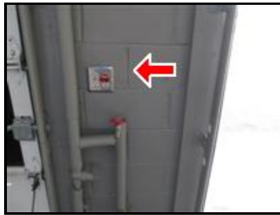
3.2 Picture 2 No Power - Shop
