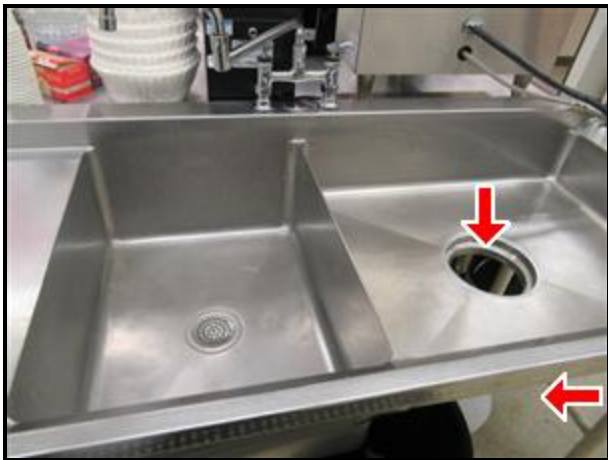
K. Picture 5 Opening / Disposal Missing
