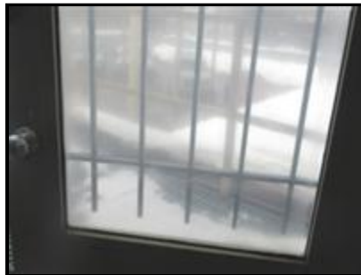
B. Picture 10 Failed Thermal or Dirty
