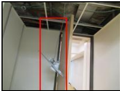
I. Picture 1 2nd Floor Light Fixture
