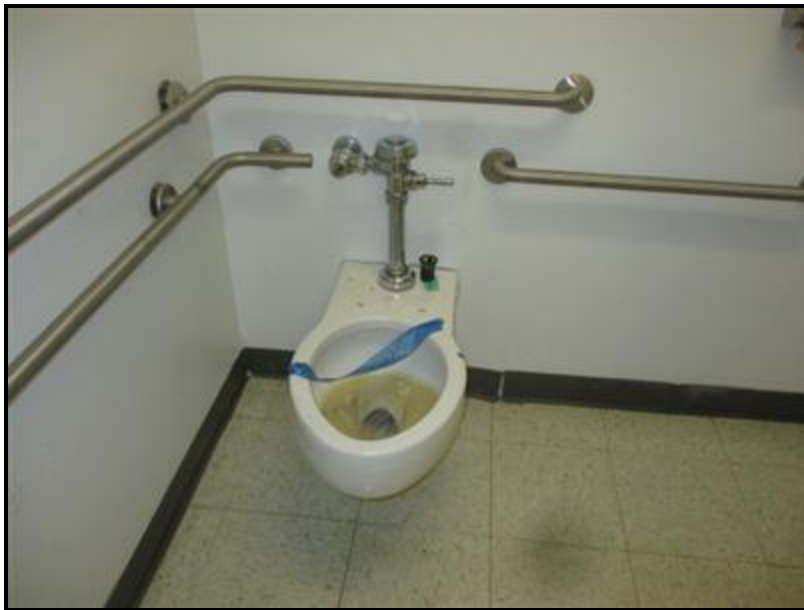
E. Picture 12 Leaks / No Seat
