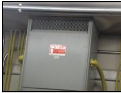
I. Picture 8 Transformer
