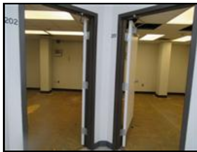
A. Picture 17 2nd Level - Missing Floor Covering
