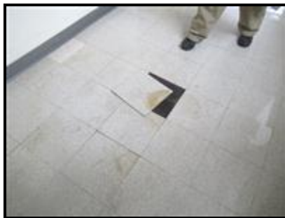
A. Picture 11 2nd Floor Loose Tile
