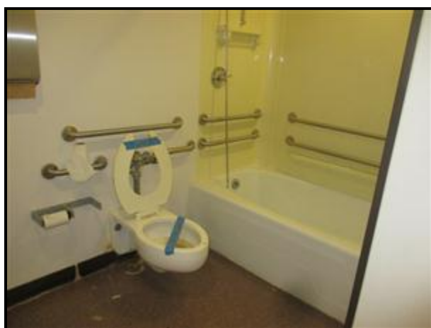
E. Picture 3 Tub Room / Leak / Broken Seat
