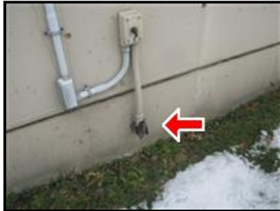
I. Picture 10 Exposed Wires/ Dumpster Area
