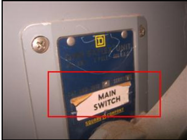
H. Picture 1 Main Switch
