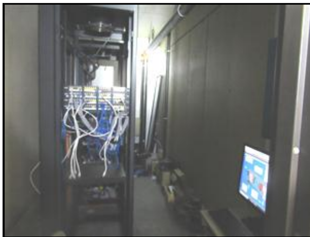
F. Picture 7 Automated Control Room
