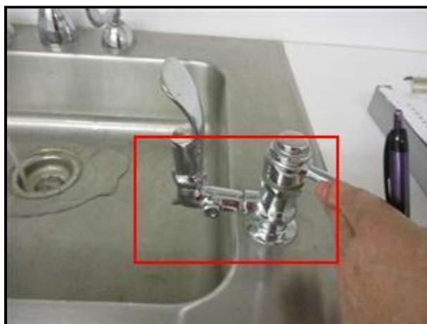
E. Picture 2 Classroom Fountain Leaks
