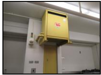
I. Picture 9 Kitchen Transformer Hums Loudly
