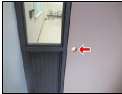
B. Picture 7 Missing Hardware
