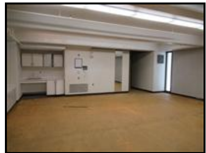
A. Picture 13 2nd Floor Missing Floor Covering
