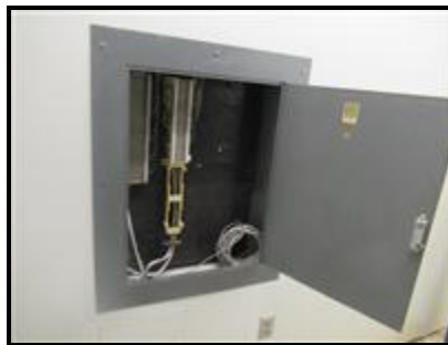
E. Picture 4 Low Voltage
