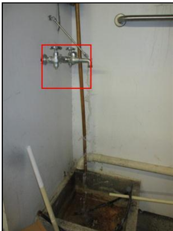
E. Picture 1 Mop Sink Leaks
