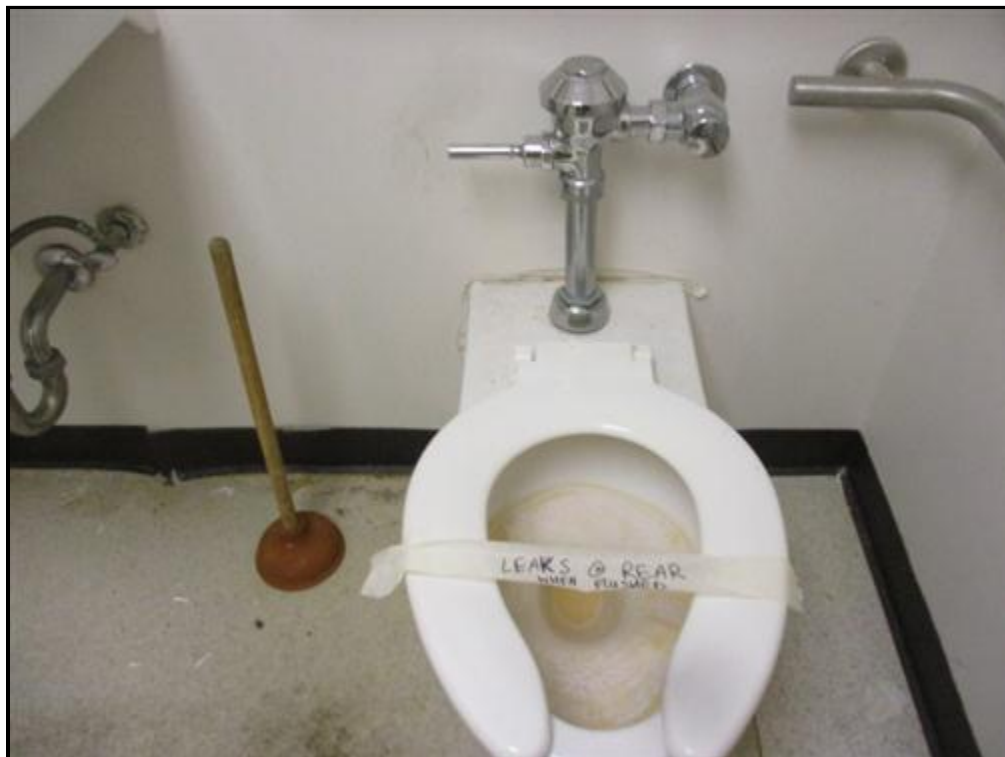
E. Picture 9 Leaks at Rear
