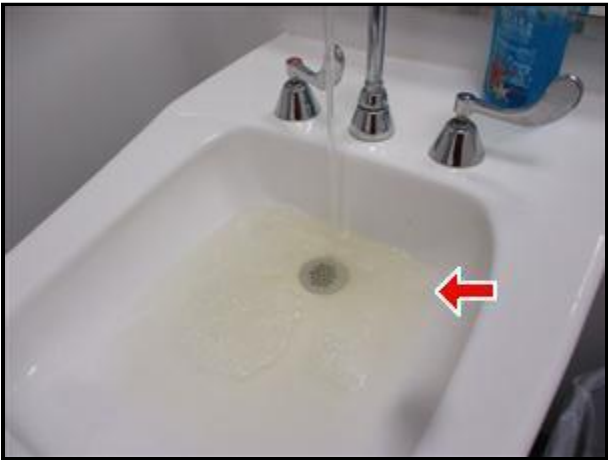
E. Picture 17 Clogged / Slow Draining
