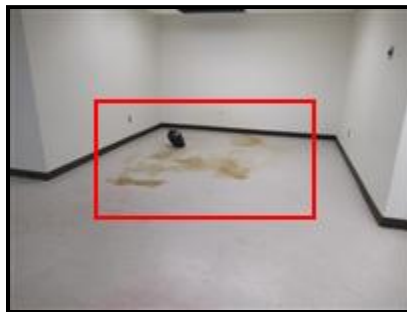
A. Picture 12 2nd Floor Water Stained
