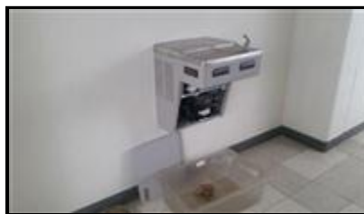
A. Picture 5 Not Working 2nd Floor
