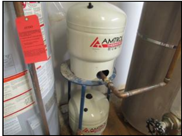
D. Picture 2 Expansion Tanks
