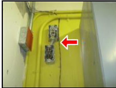
I. Picture 11 Open Electric Boxes
