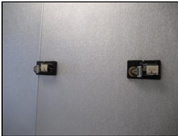
F. Picture 12 Missing Tstat Covers
