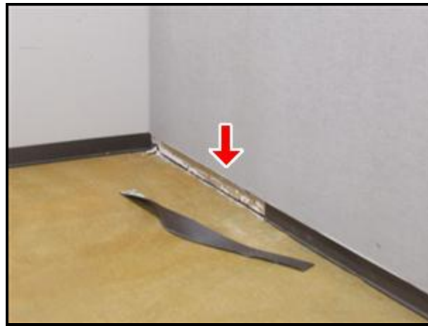
A. Picture 15 Loose Trim Missing Carpet
