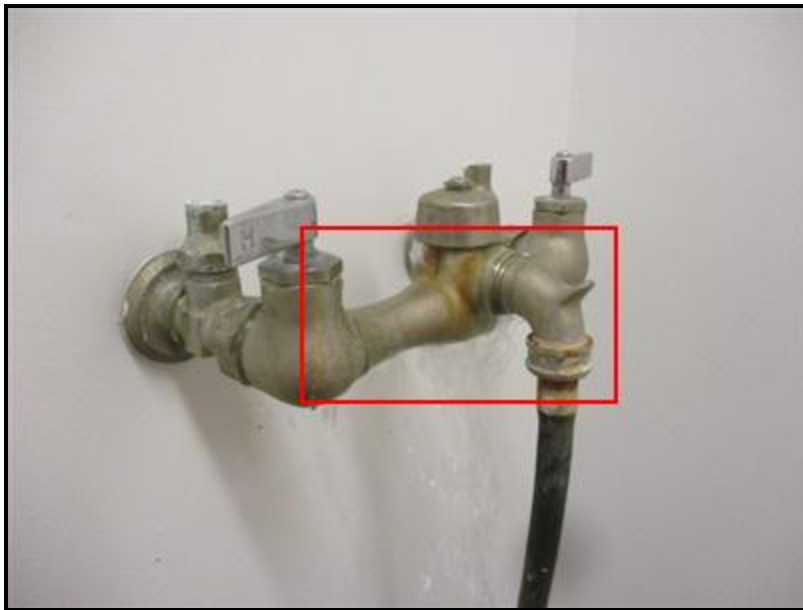
E. Picture 10 Leaks
