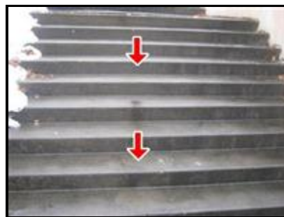
G. Picture 3 Missing Rail
