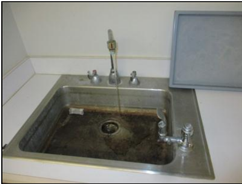
E. Picture 11 Faucet Leaks / Sink Heavily Corroded
