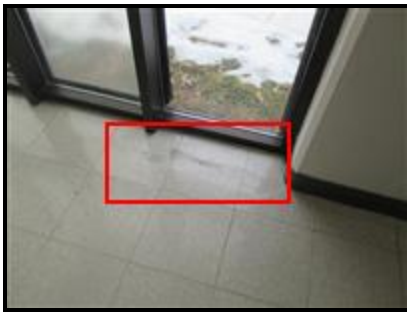
A. Picture 14 Cracked Tiles - 1st Floor
