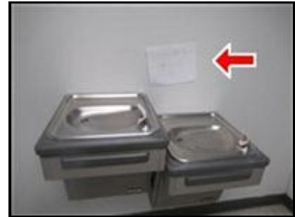
A. Picture 4 Not Working - 1st Floor
