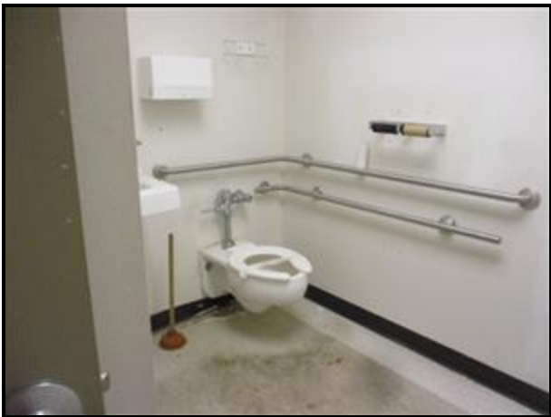
E. Picture 14 Clogged
