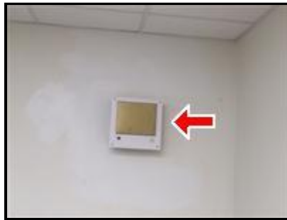
E. Picture 2 Intercom Speaker - 2nd Floor
