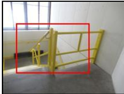
D. Picture 2 Large Gaps
