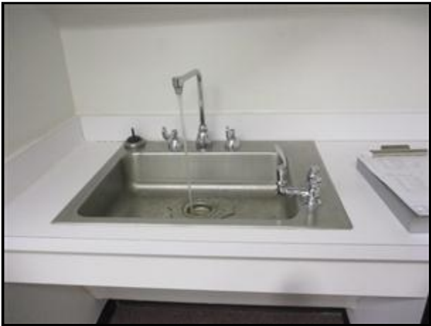
E. Picture 16 Leaks
