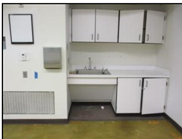
E. Picture 4 Sink Leaks
