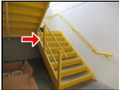
D. Picture 1 Large Gaps
