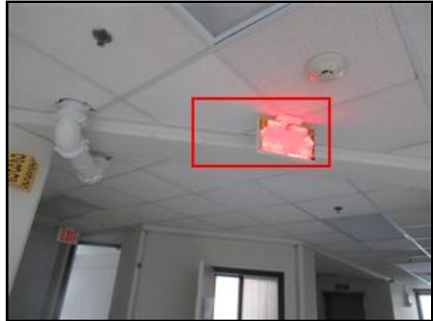
B. Picture 2 Broken
