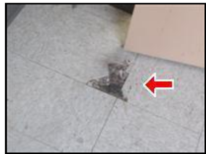
A. Picture 18 2nd Floor Damage Flooring
