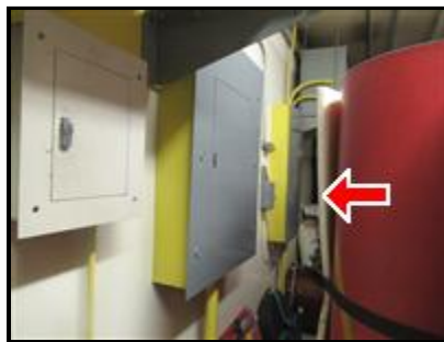
H. Picture 6 Obstructed in Gym
