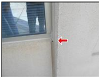
D. Picture 2 Worn Caulk
