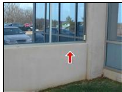
D. Picture 3 Weeps Caulked Over
