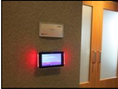
D. Picture 1 Meeting Room Screens
