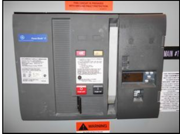
F. Picture 9 3,000amp Circuit Breaker
