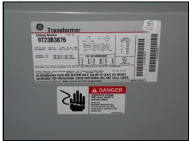
F. Picture 5 2nd Floor 150kva
