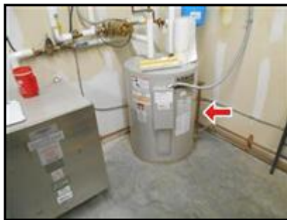
C. Picture 1 Main Level Unit
