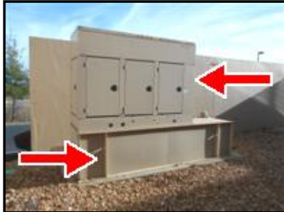
F. Picture 1 Generator Above / Tank Below
