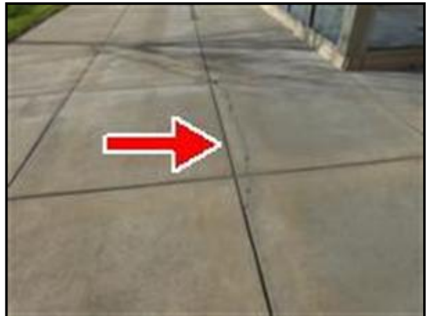
F. Picture 4 Common Cracks
