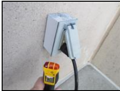
G. Picture 1 Defective Outside GFCI
