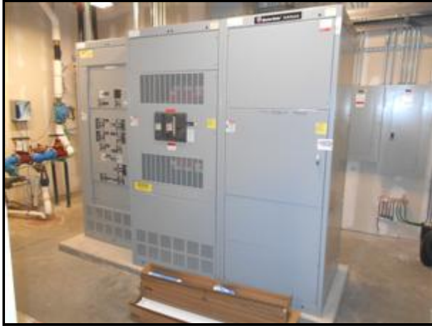
F. Picture 8 Main Panel Housing
