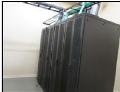
D. Picture 4 Computer Room Servers
