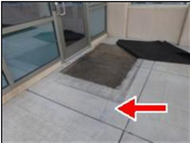
F. Picture 3 Sample Minor Cracks
