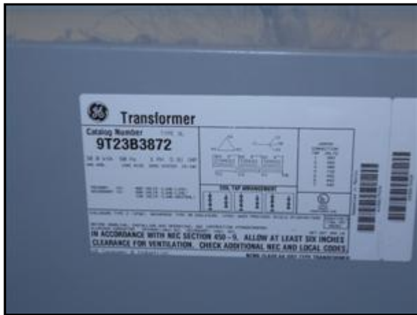
F. Picture 4 1st Floor - 30kva
