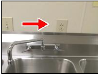
G. Picture 2 Not GFCI
