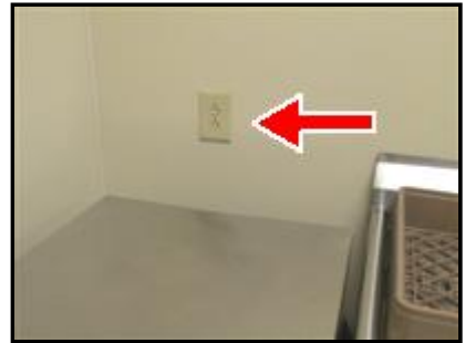
G. Picture 3 Not GFCI
