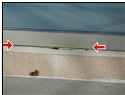
D. Picture 1 Worn Caulk
