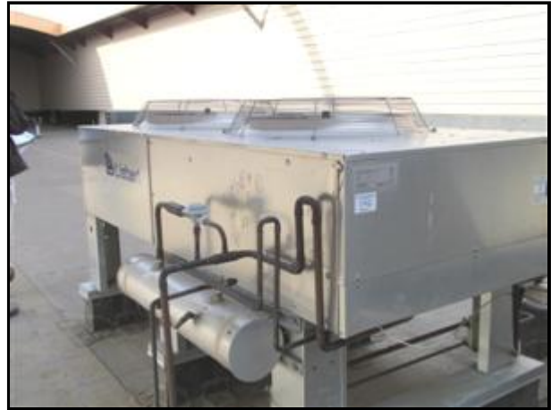
E. Picture 7 Liebert Condensor
