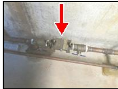
11.3 Picture 4 Backflow Device
