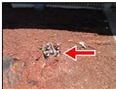
4.3 Picture 7 Exposed Outside Electrical Wires
