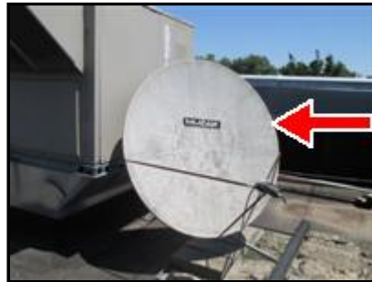
11.3 Picture 3 Rooftop Dish
