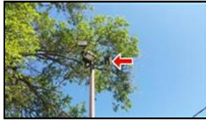
4.3 Picture 1 Pole Lights
