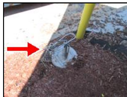
4.3 Picture 8 Exposed Outside Electrical Wires
