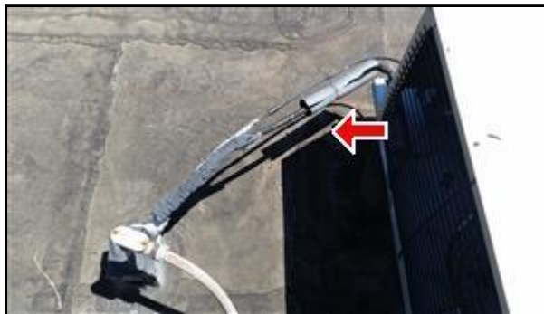
3.3 Picture 5 Missing Insulation
