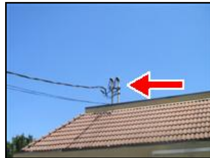
4.0 Picture 2 Overhead Service Entry Wires
