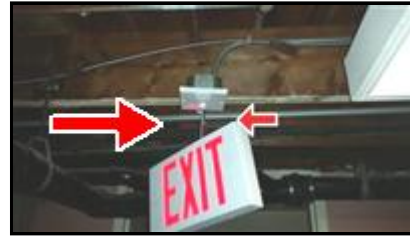
4.3 Picture 2 Exit Sign Dangling by Wires
