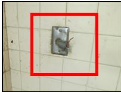
4.3 Picture 5 Bare Exposed Wire Ends
