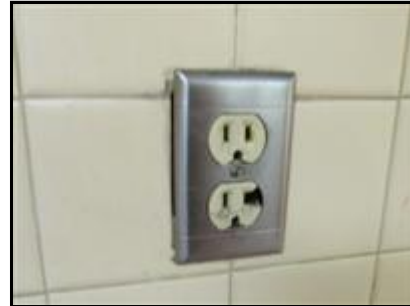
4.3 Picture 4 Sample Damaged Outlets
