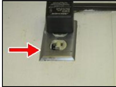
4.3 Picture 9 Damaged Outlet
