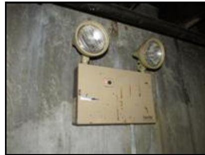
4.3 Picture 6 Lights Not Working
