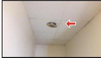
4.3 Picture 3 Loose Can Lights
