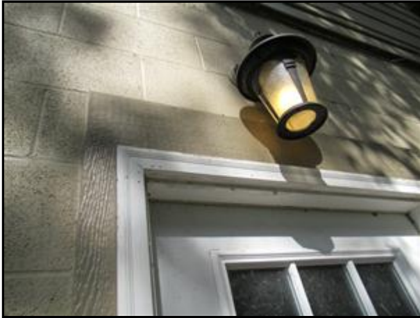
9.2 Picture 1 No Flashing Seen
