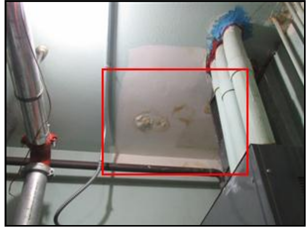
11.1 Picture 8 Moisture Stain Mechanical Room
