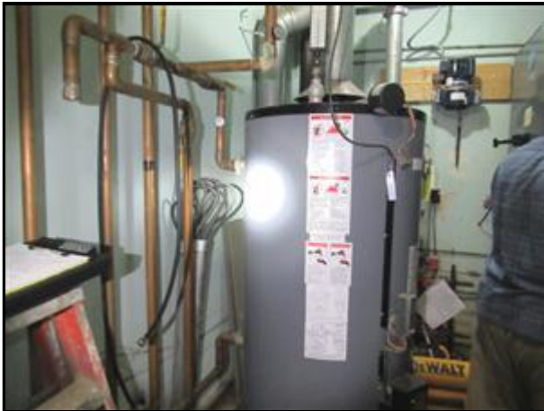
3.5 Picture 1 Water Heater
