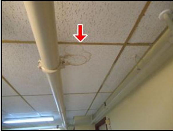
11.1 Picture 7 Moisture Stain Main Level
