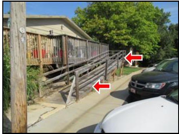
6.5 Picture 8 Loose Rails
