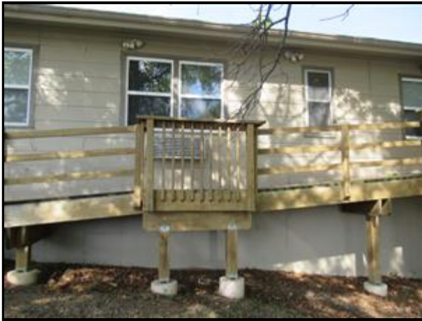
6.5 Picture 1 Large Gaps in Rails
