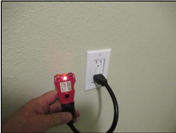
4.2 Picture 1 Ungrounded / Defective GFCI
