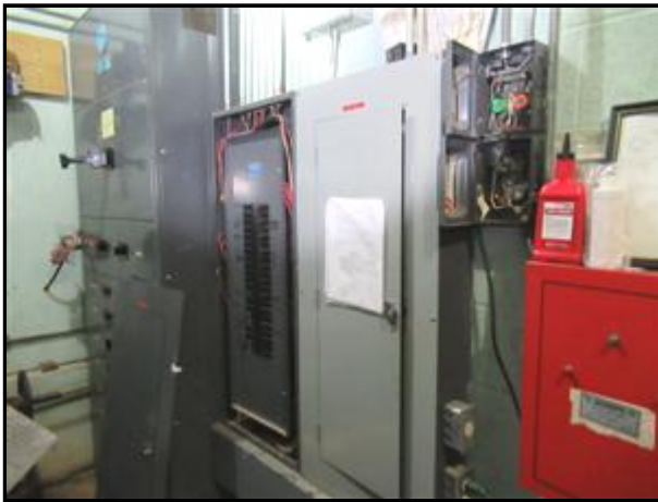
4.1 Picture 1 Main Panel & Sub-Panels
