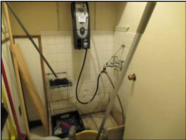
1.0 Picture 6 Mop Sink
