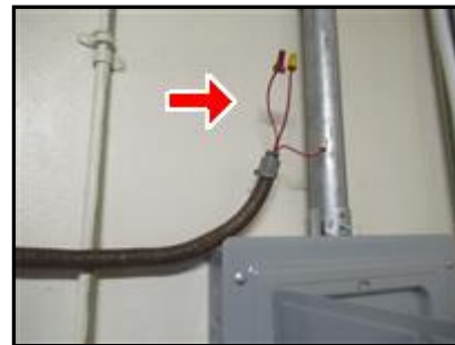
4.2 Picture 4 Exposed Splices
