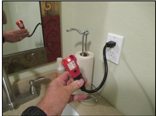
4.2 Picture 2 Ungrounded / Defective GFCI
