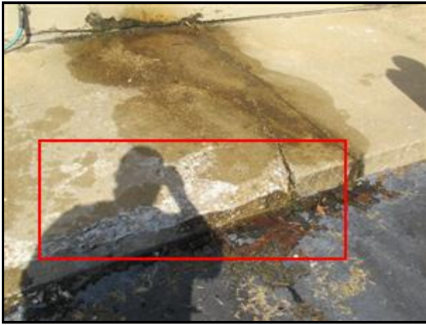
6.1 Picture 1 Damage / Trip Concern
