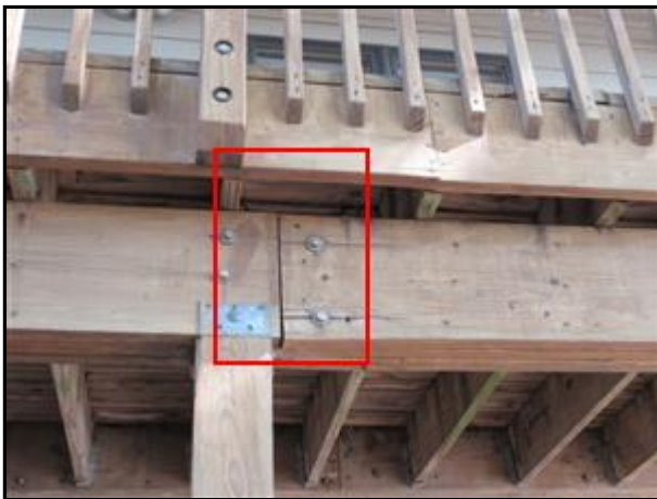
6.5 Picture 3 Joists Not on Support Post
