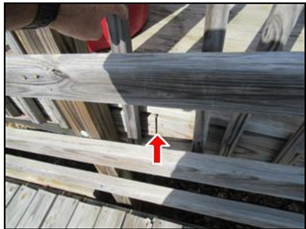
6.5 Picture 10 Big Gaps
