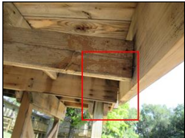
6.5 Picture 6 No Joist Hangers
