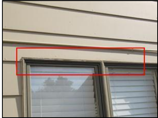
9.2 Picture 2 Head Flashing Not Seen
