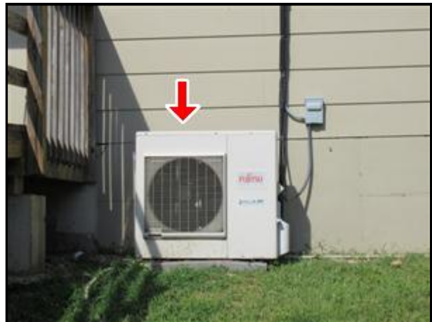
5.0 Picture 6 Split System Fujitsu
