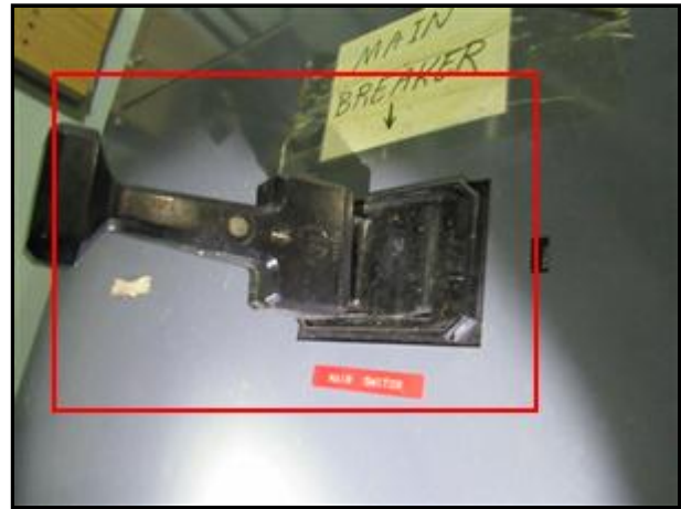
4.1 Picture 2 Main BReaker
