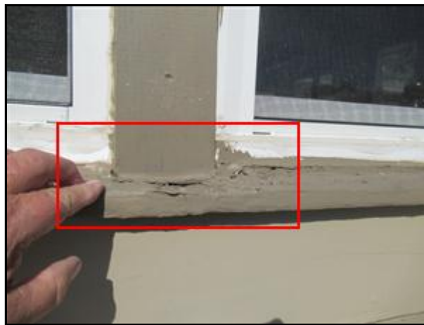
9.1 Picture 9 Window Sill
